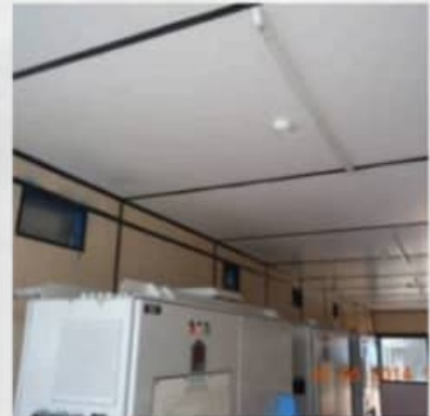
Electrical Panel Cabin
